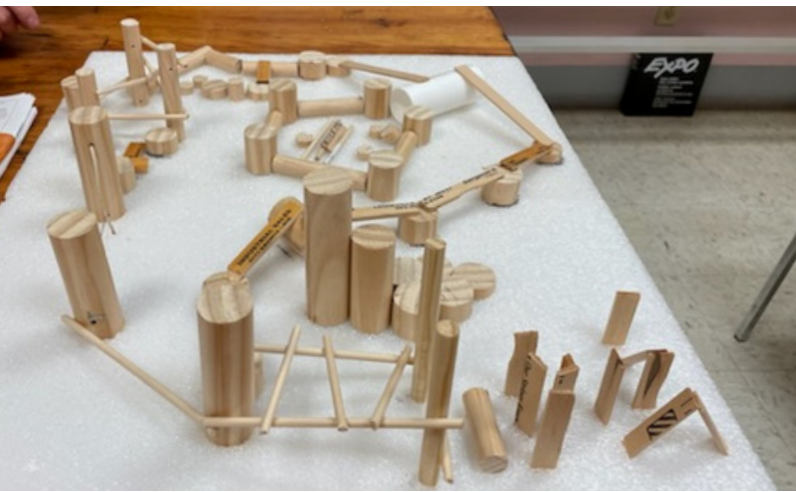
Left, top: A preliminary model of the nature play area. Below: Lauren Hendrickson attaches footholds to a climbing wall.
